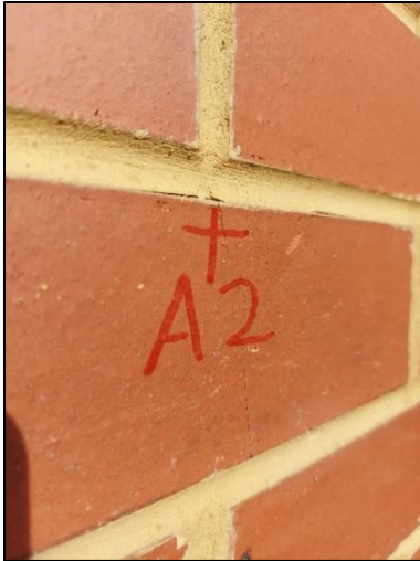
Photograph No. 4 – Damage caused following impact at location B2 Blue Zone
