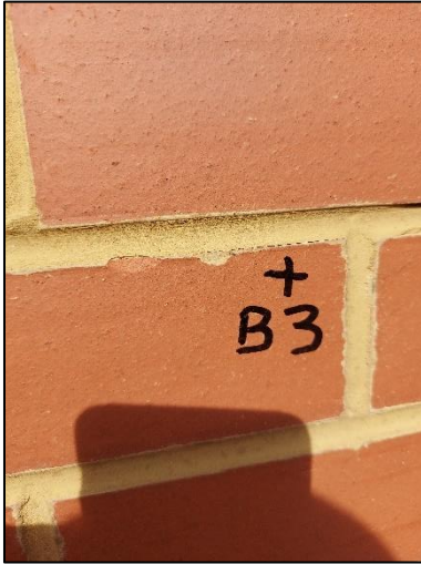
Photograph No. 8 – Damage caused following impact at location A2 Red Zone
