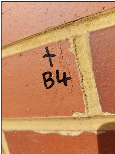
Photograph No. 6 – Damage caused following impact at location B4 Red Zone
