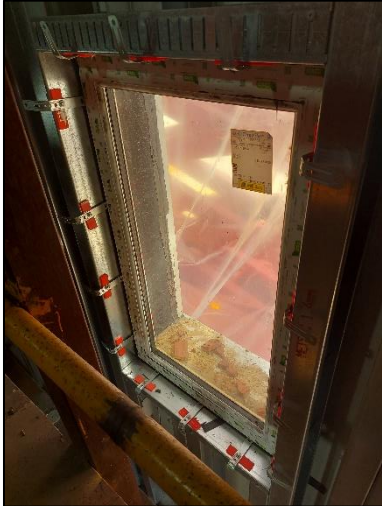
Photograph No. 16 - Sample with bricks partially removed
